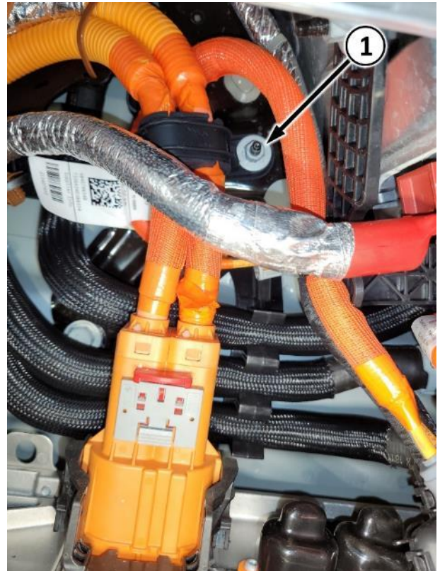
Figure 43 – HV Battery - Primary
